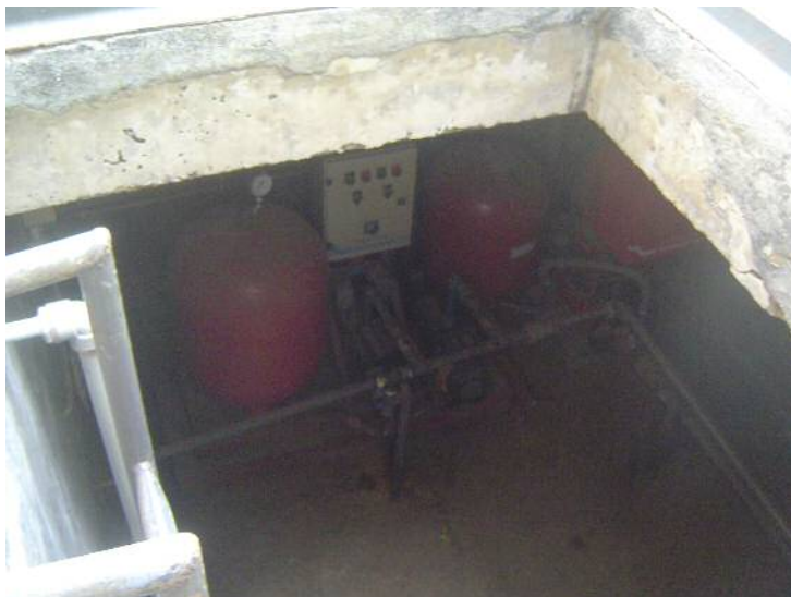
Water Supply Metering Chamber
