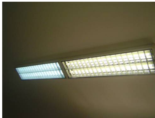
Existing four-foot 2-lamp fluorescent Fixture
