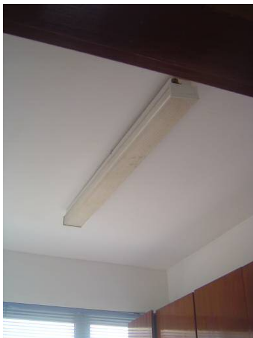
Existing 1-lamp Wrap-Around Lighting Fixture
