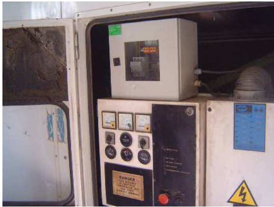
System Control Module of the Standby Power Generator
