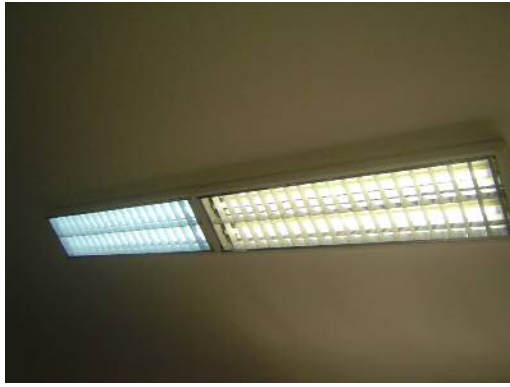
Fig 7.1 - Existing Lighting System – F40T12
