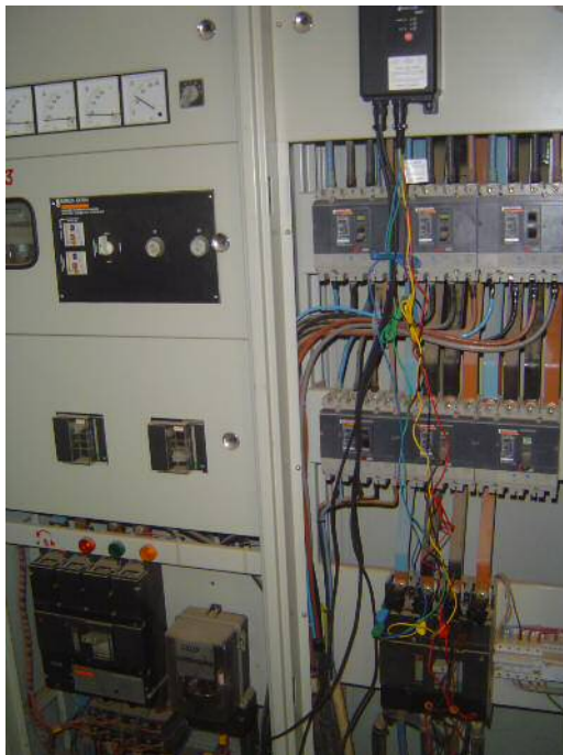
Installed Power Analyzer at the Power Monitoring Period
